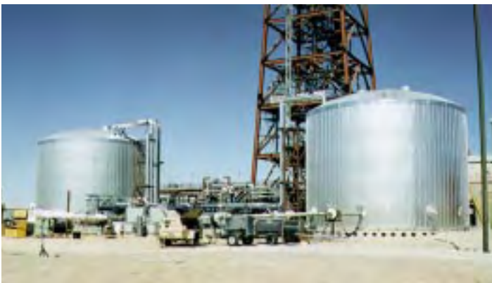
Storage is the key to molten-salt power towers. These two tanks provide three full hours of storage at Solar Two.
